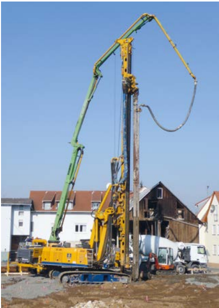
BF 13, ROB, Deutschland BF 13, VCC, Germany
